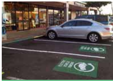
IMAGE 2. MILILANI, HI THE EVSE IS MOUNTED ON AN EXISTING POST AS TO NOT SHORTEN THE PARKING SPACE OR INTERFERE WITH PEDESTRIAN ROUTES.
