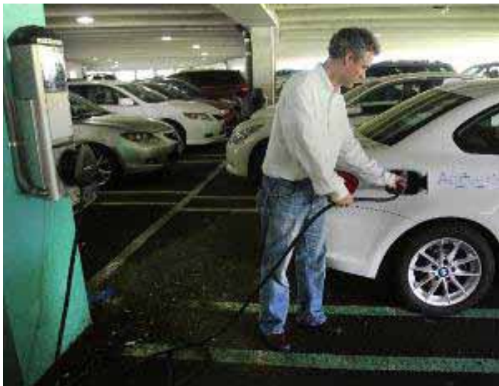
IMAGE 4. PARAMUS, NJ BY MOUNTING THE EVSE ON AN EXISTING POST BETWEEN SPACES, PARKING SPACE SIZES ARE MAINTAINED AND WHEEL STOPS OR BOLLARDS DO NOT NEED TO BE INSTALLED
