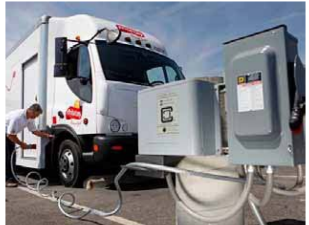
IMAGE 7. FRITO LAY MOST TRUCKS USE THE J1772 STANDARD CONNECTOR TO CONNECT TO EVSE.
