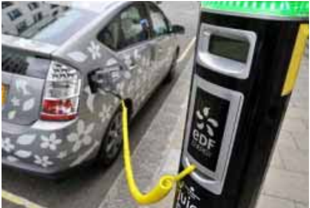
IMAGE 5. LONDON, UK CORD MANAGEMENT TECHNOLOGY AND EVSE PLACEMENT IS ESPECIALLY IMPORTANT FOR ON-STREET PARKING SO AS TO NOT CREATE TRIPPING HAZARDS. EVSE SHOULD NOT BE PLACED IN A LOCATION THAT WOULD CROSS SIDEWALKS OR PEDESTRIAN PATHS. RETRACTION DEVICES OR A PLACE TO HANG PERMANENT CORDS AND CONNECTORS SUFFICIENTLY ABOVE THE GROUND SHOULD BE PRESENT ON ALL EVSE.
