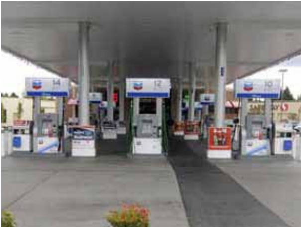
IMAGE 6. BEAVERTON, OR THE EVSE IS INTEGRATED INTO EXISTING INFRASTRUCTURE. IT IS LOCATED BETWEEN OTHER GAS PUMPS AS TO NOT BLOCK TRAFFIC SINCE THE CHARGING VEHICLE MAY BE PARKED FOR UP TO HALF AN HOUR.
